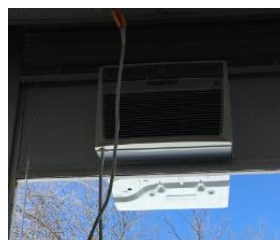
Figure 14 - Typical Window AC Unit
