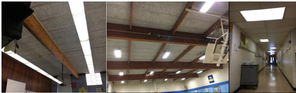
Figure 10 - Lighting Fixtures with Lenses in Poor Condition
